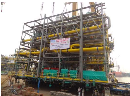
CdM CO 2 Gas Compression Module
