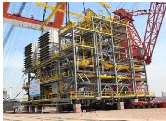
CdM Power Generation Module
