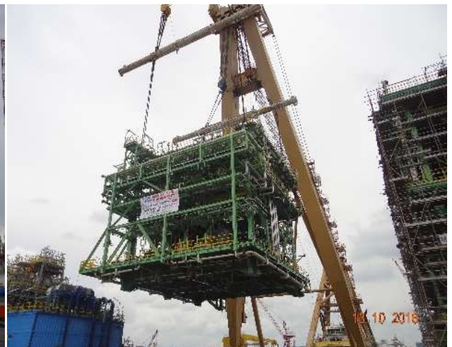
Export Gas Compressor Module
